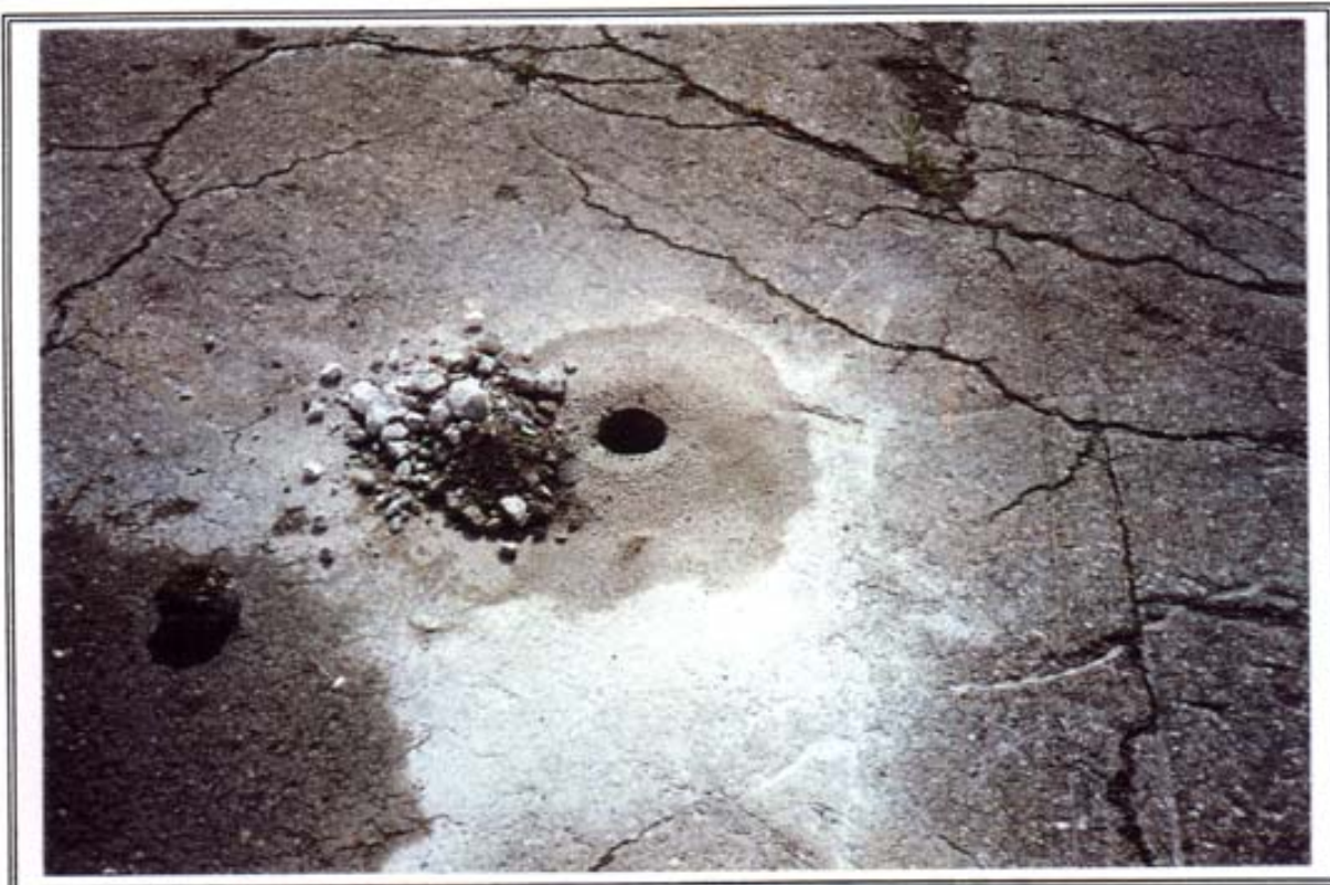
PHOTO 20. 240 VULCAN STREET: Study Area C - View of Core Boring Through Concrete Slab (Core C-3).
